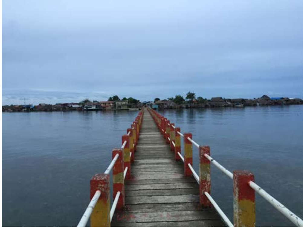
A 165m pedestrian bridge that connects the community of Playón Chico to the mainland. The picture was taken coming from the mainland to the island. Photo by Carlos Arenas.
